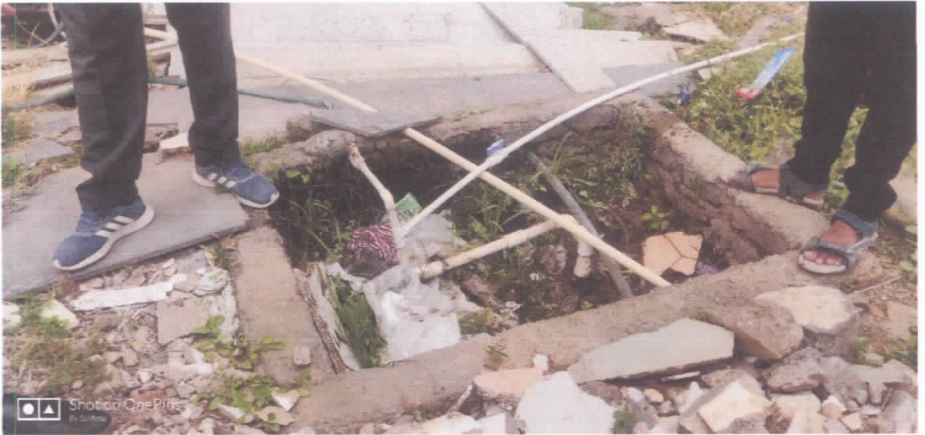
M/s Jubilee Park – Bore well
